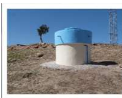
Station de relevage
